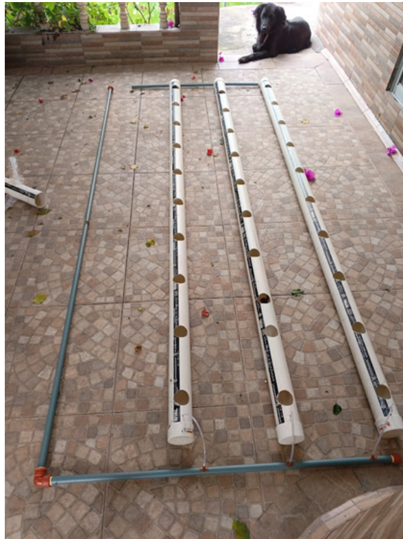
Figure 9. Irrigation Piping System
