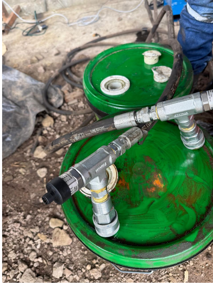
Fig. 9. Pressure transducers installed in the hydraulic lines during commissioning
