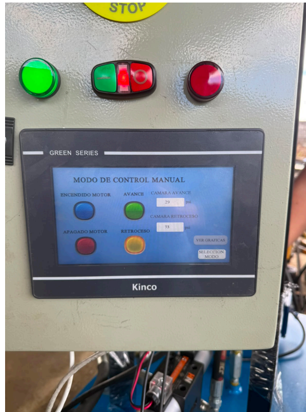
Fig. 11. HMI during manual-mode commissioning and pressure verification
