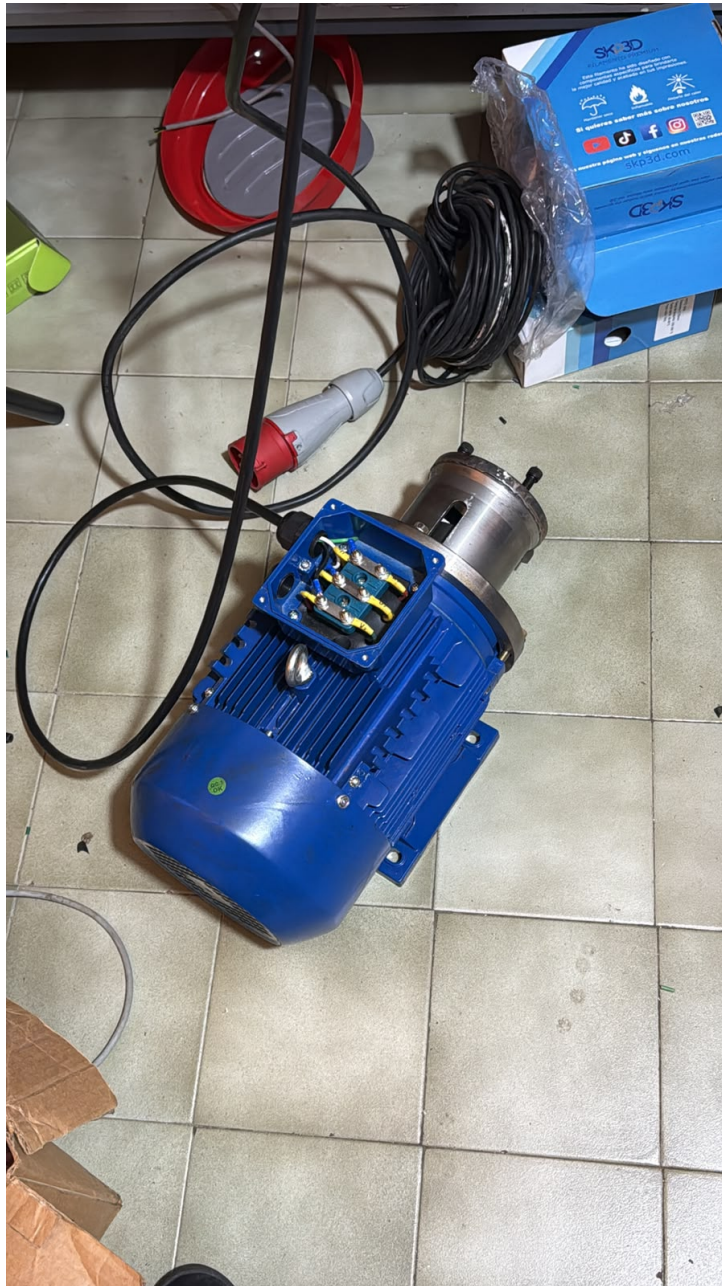
Fig. 6. 5.5 hp three-phase motor in a delta configuration
