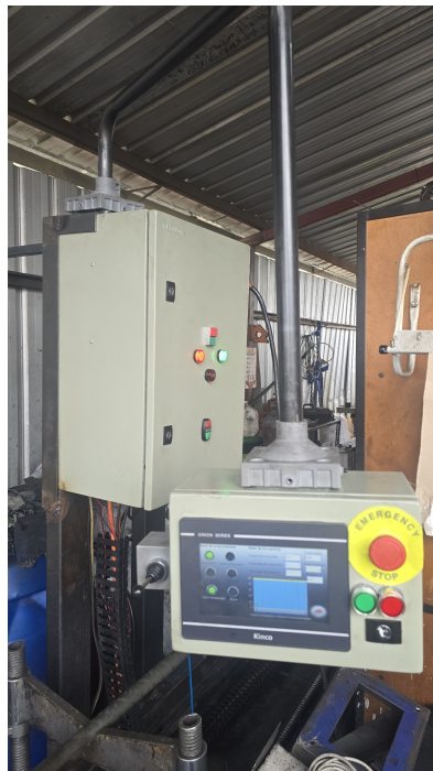
Fig. 16. Relocated operating panel with HMI, physical buttons, and joystick.
