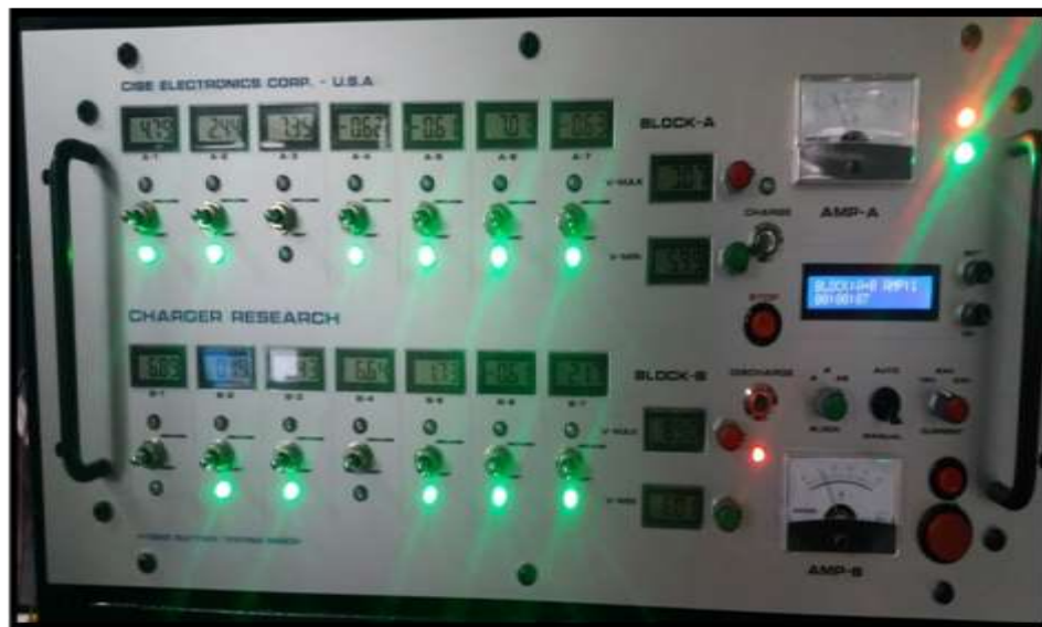
Figura 46. Panel de control encendido (Cise Electronics)
