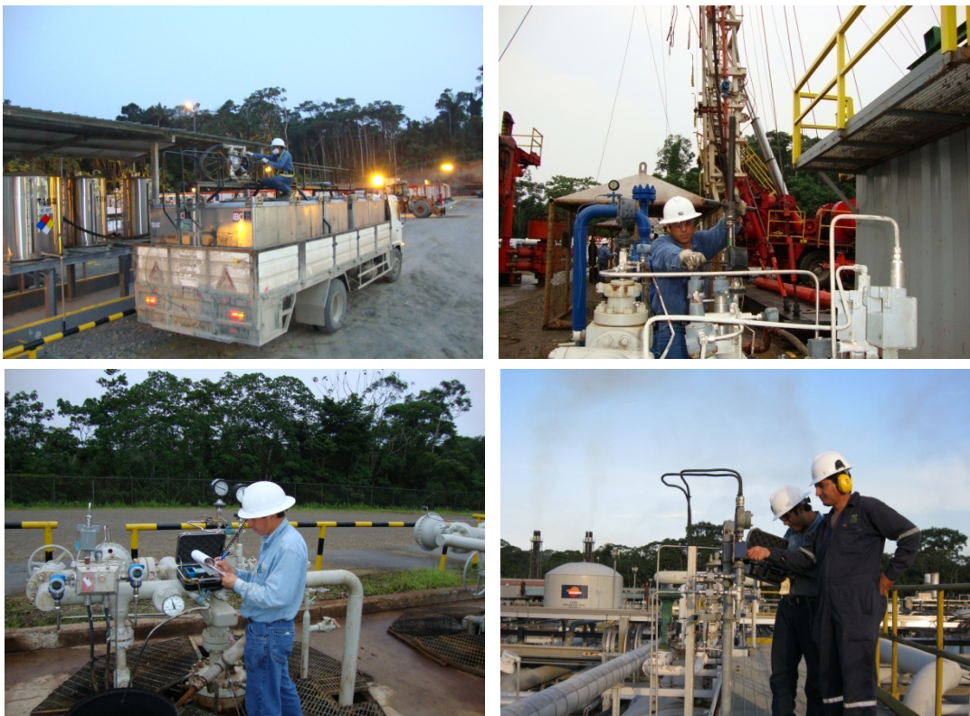
Figura 26. Servicios "in situ" Oil Field Chemicals
